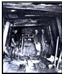
Above: Photograph part of Mildenhall collection in National Australian Archives. It shows work in the sewer tunnel. The man second from the right and the only dry person in the photograph is Jeremiah Dillon.
